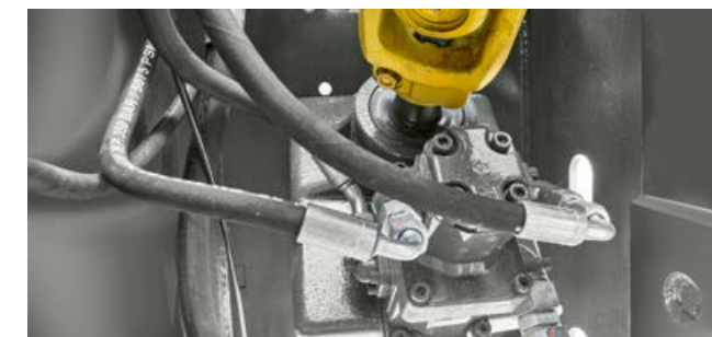
Two oil pumps supply hydraulic oil to the input transmission and the TURBO FAN knotter cleaning system.
